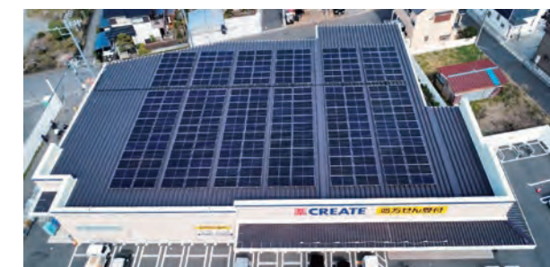
Solar panels installed on store rooftop
